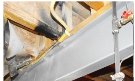
Floor support burned by ruptured CSST
